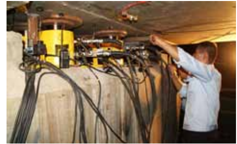
TLP General Purpose Cylinders with tilt saddles are lifting the bridge deck in pier reconstruction.
